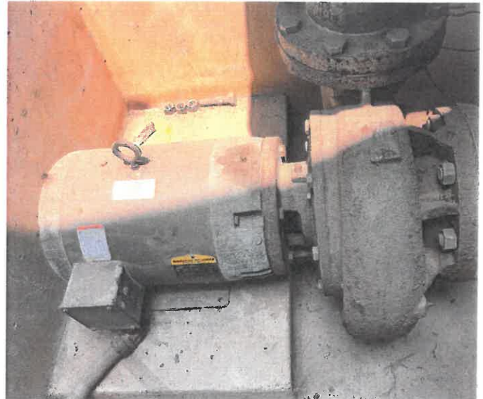
Aging Water Slide Booster Pump and Motor
