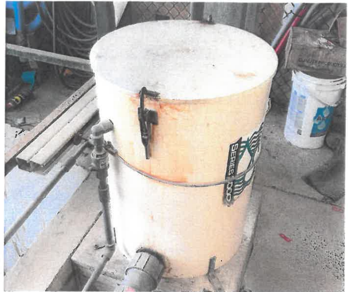
Chlorine Tablet Erosion Feed System
