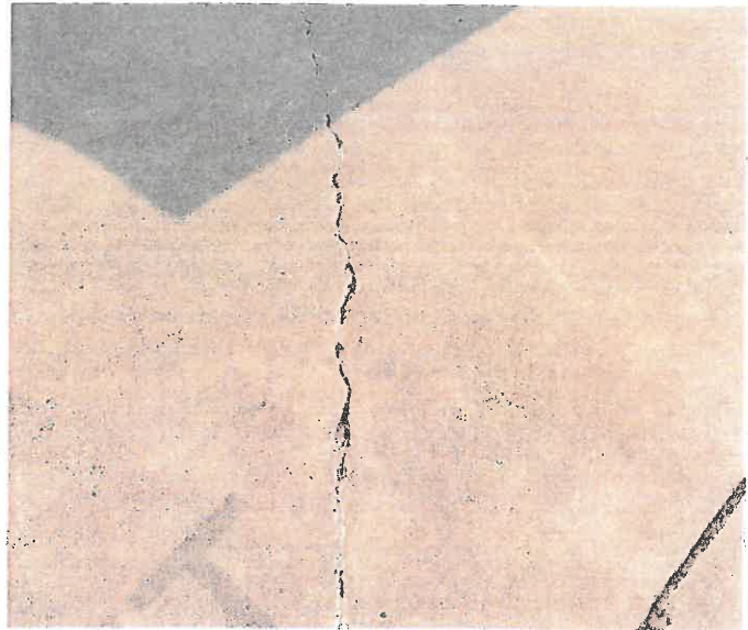
Crack in Pool Deck
