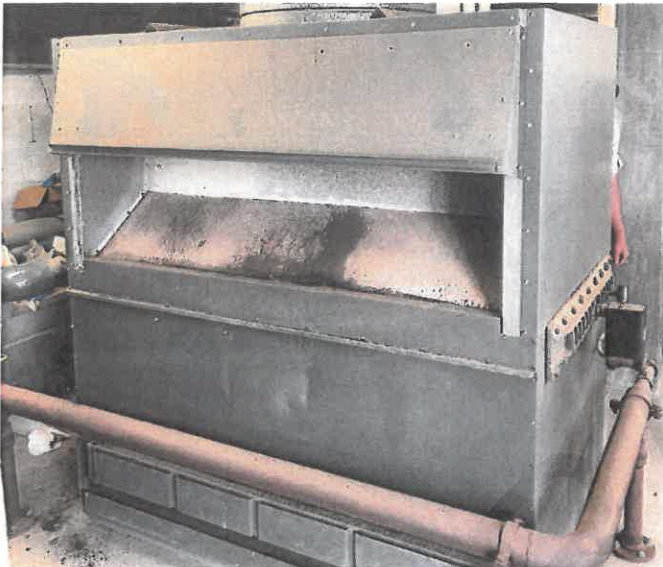
Existing Heater for Swimming Pool
