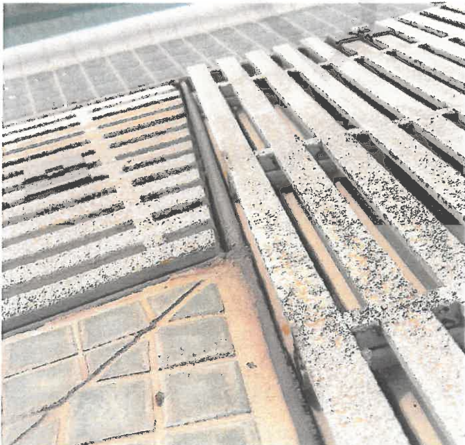
Gutter Grating Popping Up
