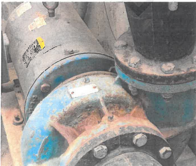
Aging Circulation Pump and Motor
