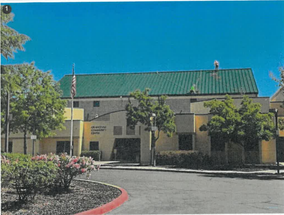
1 Crew is installing the downspouts, running the seamer on the panels and finishing up the roof!
