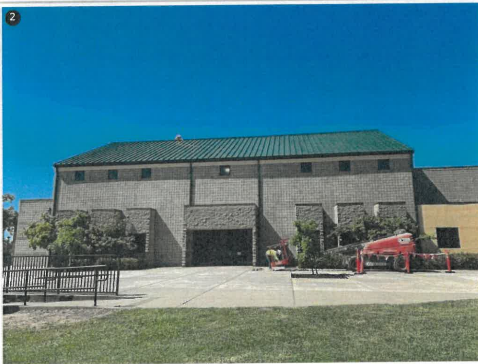
2 Back of the roof. Project turned out fantastic, great job by D7 crew!
