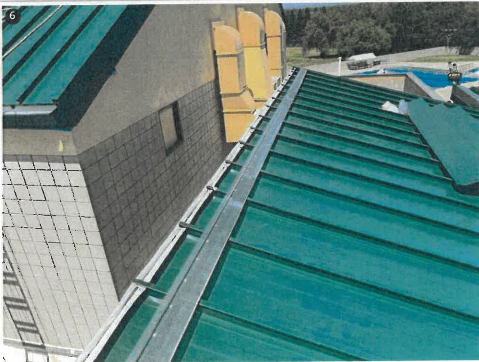
6 The vent is covering the head closures, but they are installed in every panel. You can also see the top of the panel is turned up. This prevents any moisture from being blown in and getting behind the panel.
