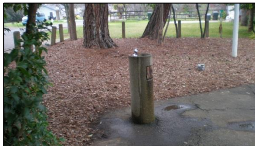
Figure 65 - Leaking Water Fountain at Lifecycle 3
