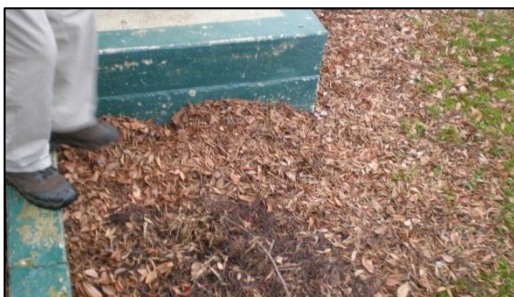
Figure 69 - High Step Safety Hazard for Pedestrian Circulation
