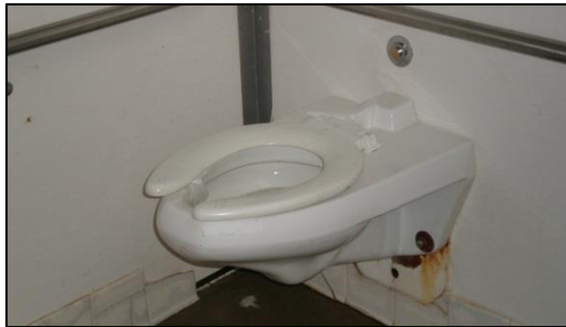
Figure 56 –Leaking Toilet and Broken Tiles
